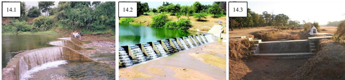
Picture 14. The sample of concrete check dams in India as constructed to slow the water flow of natural rivulets and streams. 14.1 and 14.2). At Gujarat 14.3). At Pachmarhi Hill Station
