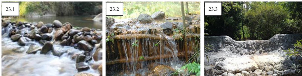
Picture 23. The check dam in Thailand is constructed using local material following as 23.1).Arrangement with rock 23.2).Rock framed with wood 25.1).Concrete framed fill with rock Source: The Office of Public Relations Region 2, 2011, Matchon online, 2008 and Parichat, 2012.
