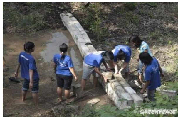
Picture 27. The sample of Solar Generation volunteers constructs a check dam in rural area.
