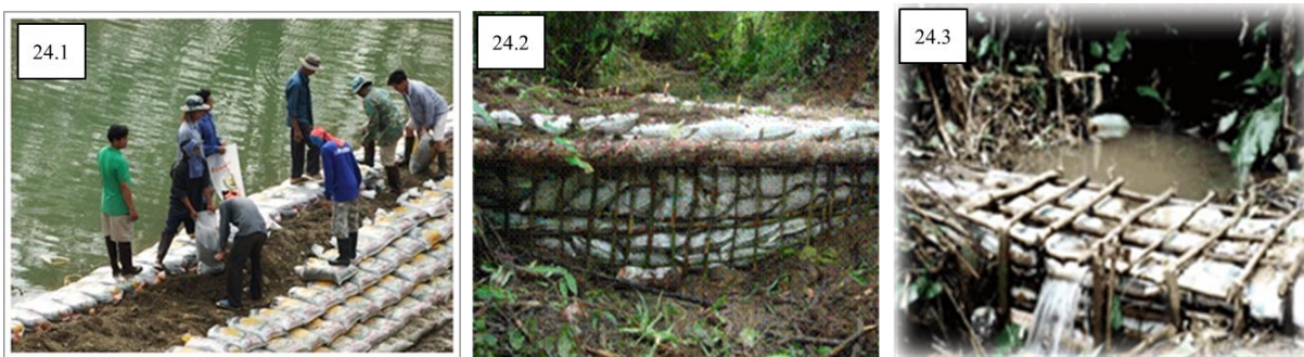
Picture 24. The check dam in Thailand is constructed using local material following as (Continued) 24.1).Sand bag arrangement 24.2).Pig-pen filled with sand bags 24.3).Sand bags framed with wood Source: Royal Irrigation Department, 2013, Hydro and Agro Informatics Institute, 2012 and Department of National Parks, Wildlife and Plant Conservation, 2012.
